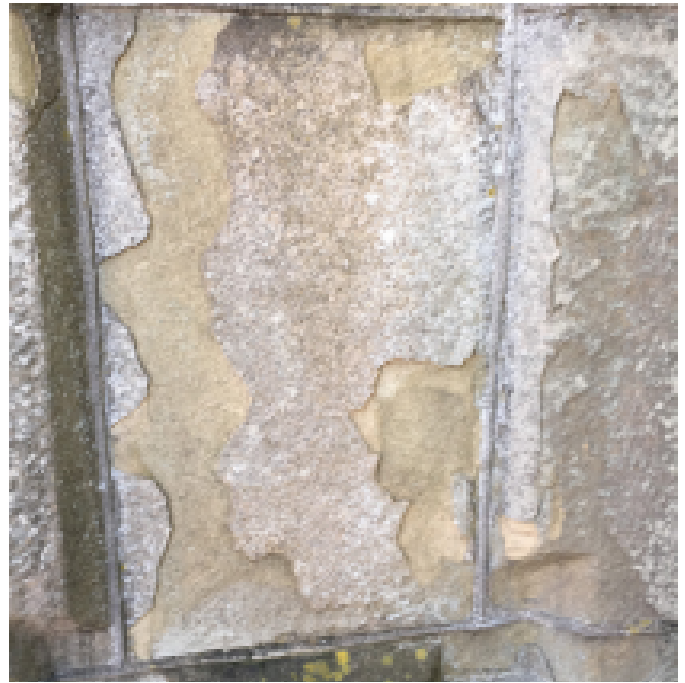
Extensive peeling at vertical surfaces of pier - including smooth and tooled surface finishes.
